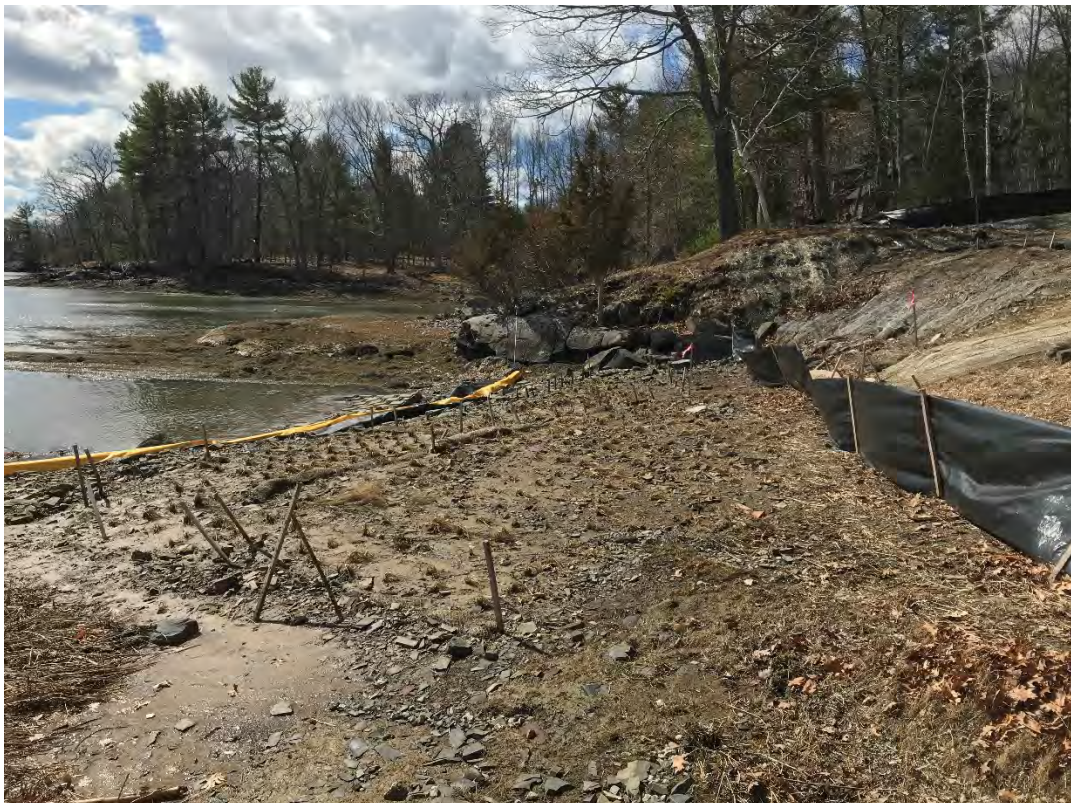
Fig 4: Toe of the slope and salt marsh restoration at the Eversource property/west side of the bay. Viewing south. (03-29-21)
