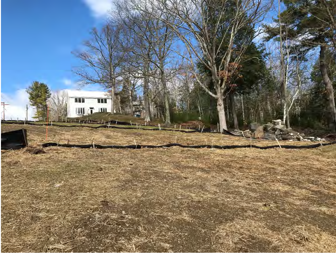
Fig 3: Slope above the cable house at the Eversource property/west side of the bay. Viewing northwest. (03-29-21)
