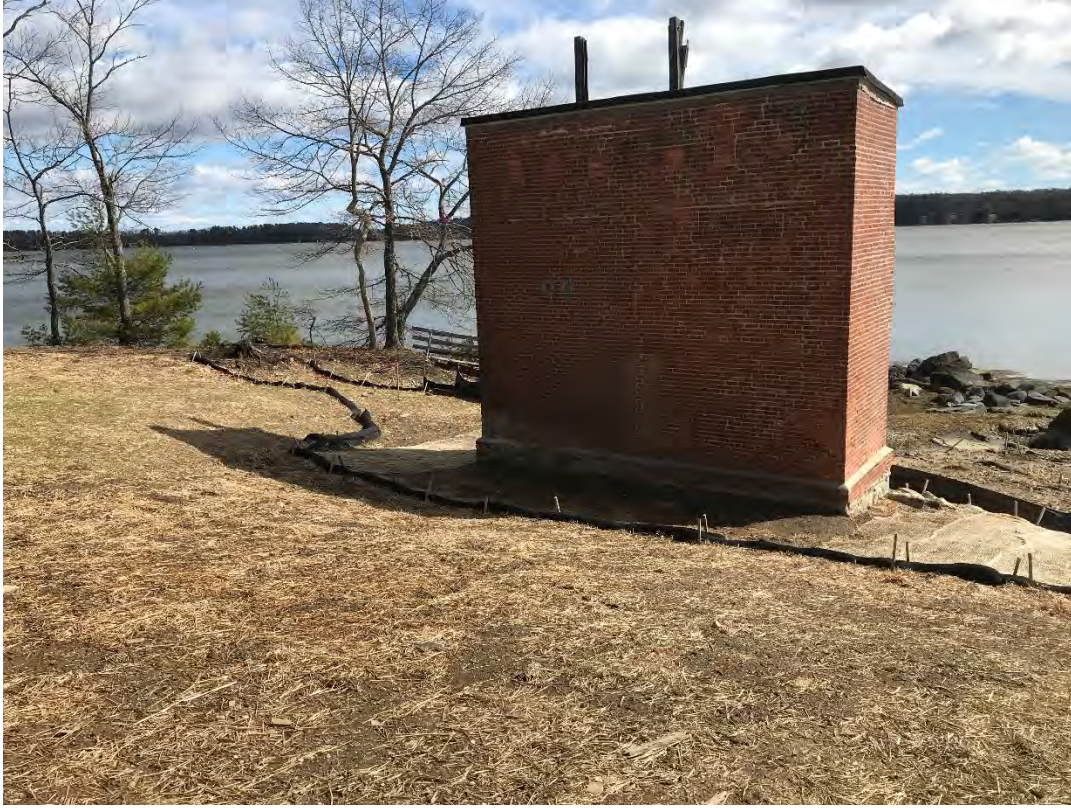
Fig 1: Slope leading down to cable house and salt marsh restoration at the Eversource property/west side of the bay. Viewing northeast. (03-29-21)
